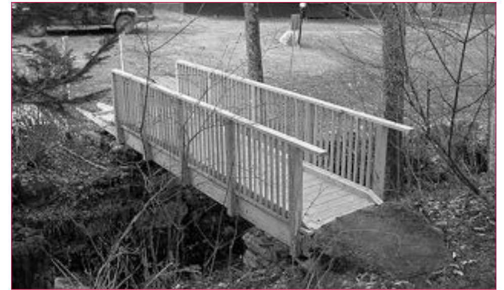
Our new wheelchair accessible bridge to the Morrill Ice House under construction this spring
